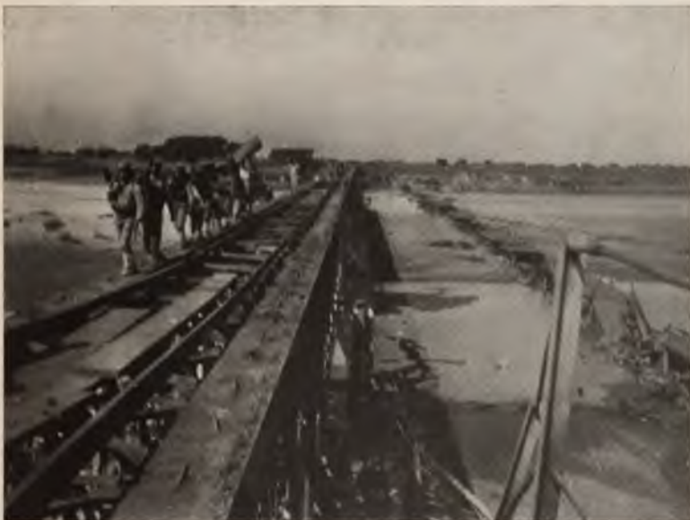
The great railway bridge at Liaoyang, partly destroyed by the Russians.
